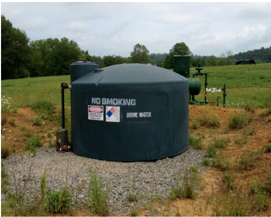
Brine Storage Tank in Pennsylvania, Photo by Nadia Steinzor
